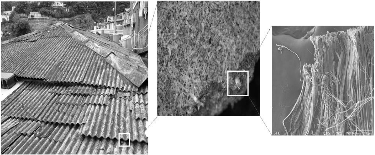
Fig. 2. Asbestos-cement slate roofs and SEM image of chrysotile in the slate roofs.
